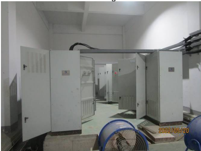
Main control room
